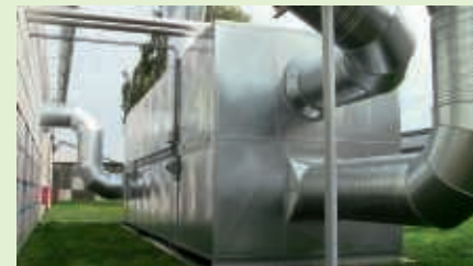
The new system for Carl Hansen & Søn is delivered with full heat recovery living up to the company's green profile.
