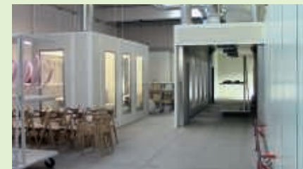
The new finishing line includes sanding booth and drying tunnel. In addition Aagaard A/S developed special trolleys for transportation of furniture into the drying tunnel.
